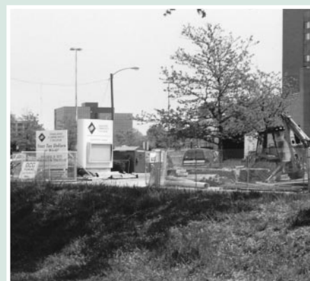
The Southfield Campus rose from under its earth berms and received a new façade and major interior renovations.
