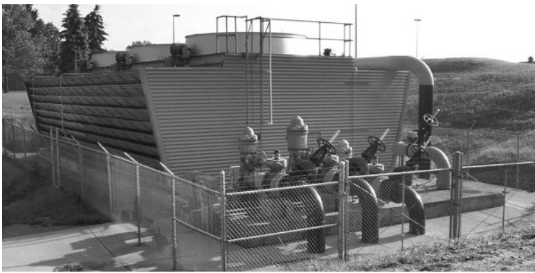
Cooling tower/chiller upgrade
