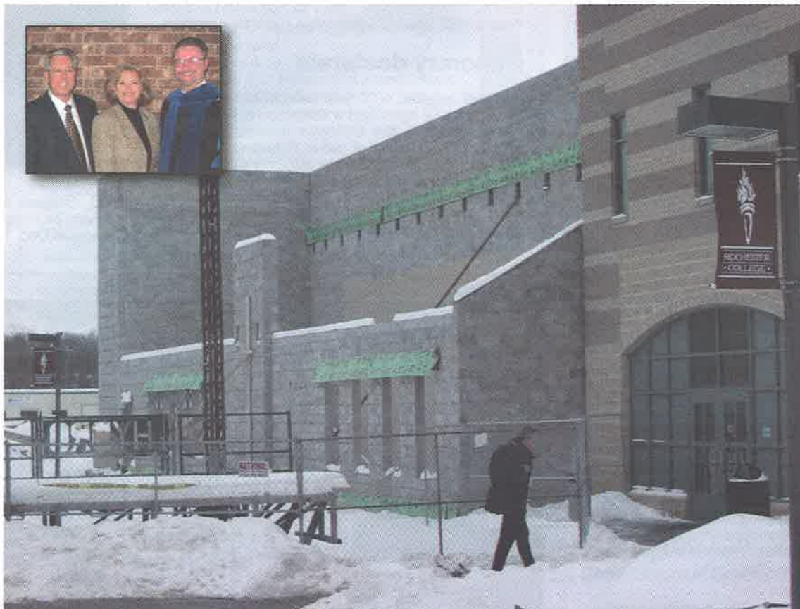
A student walks into the Ham Library (foreground) as construction continues on the student center section of the Richardson Academic Center (background). The 25,500 sq. ft. building will be home to a student center, theater/conference room, administrative suites, Academic Center for Excellence and the Department of Science. Inset: David and Patricia Richardson stand with Dr. Michael Westerfield (right), Rochester's interim president, after they announced their record-breaking $3 million commitment to Catch the Vision Phase II .
