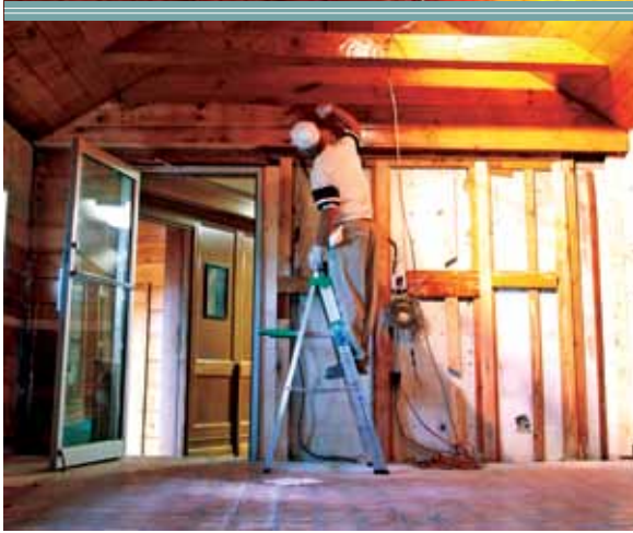
A MODEL VOLUNTEER Ron Loshier assists with the renovation of the Gallaher Center in 2009.
