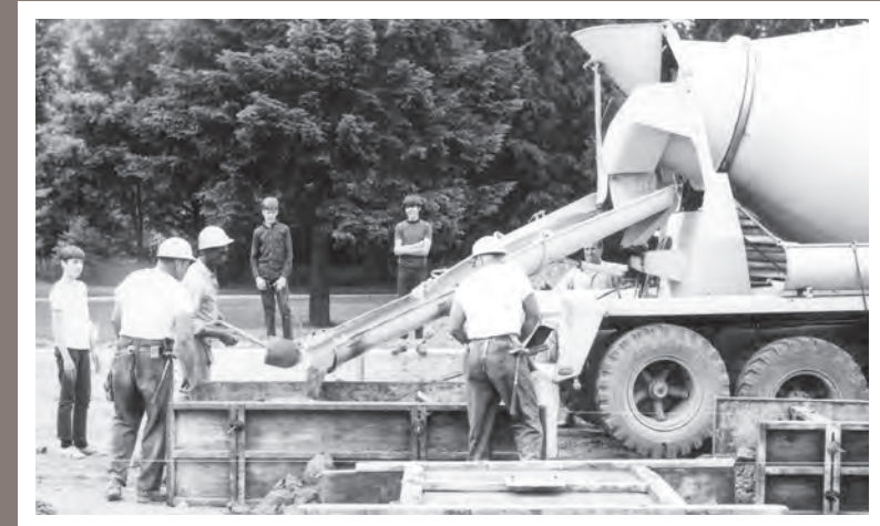
Construction workers poured concrete foundations for the Alma Gatewood Residence Hall during the summer of 1969.
