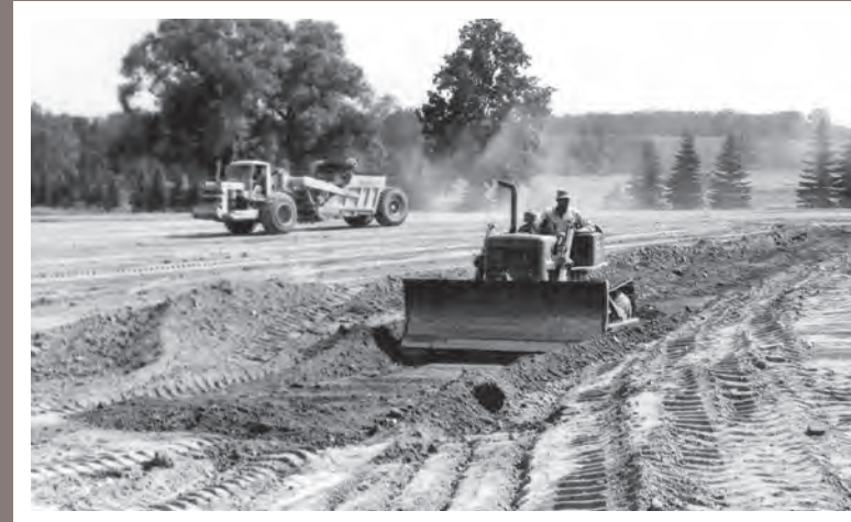
Earth moving equipment began transformation of a Gierok farm cornfield into athletic fields in the summer of 1965.
