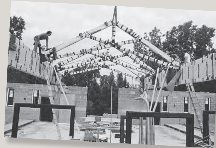
▲ Work on the chapel resumed after the end of a 1977 strike by the manufacturer of the fireproof roof decking.
